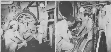
Oil Movement personnel are shown here at work on board the "Esso San Nicolas." At left, the clutch gets new shoes. At right, Henry Orman (c) gets assistance during work on cylindrical clutch drum. Supervising the job (at rear right) is Antero Gil.
